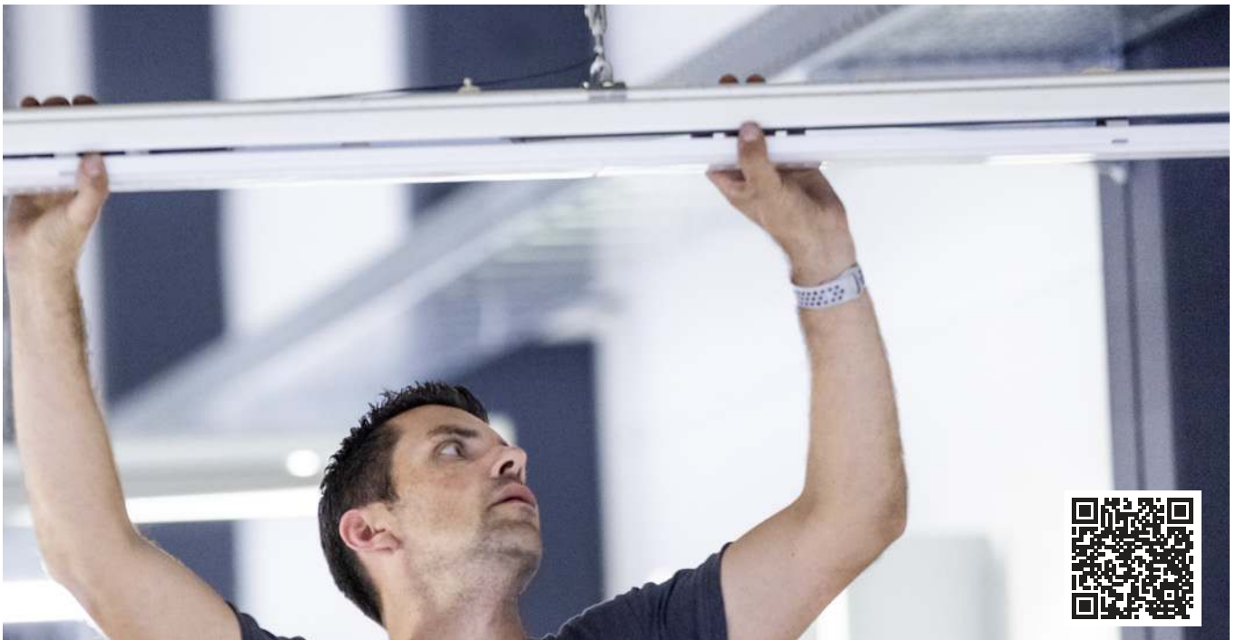
From old to new during running operation – experience the lighting refurbishment at Wache Lübeck GmbH
